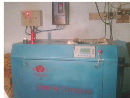
Screw air compressor
